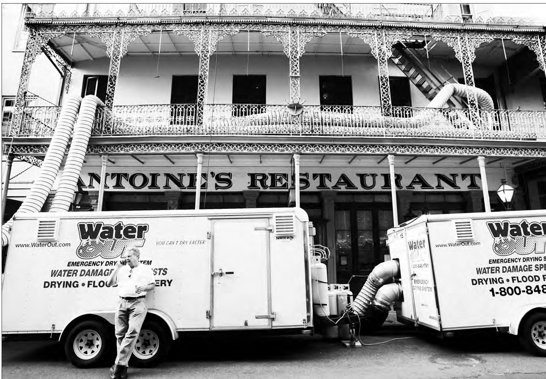
After Hurricane Katrina, Antoine’s had to pay thousands to an emergency dry-out company to pump the dank building full of dehumidified air.
