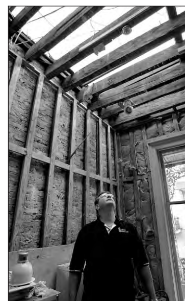
Photo for the Tribune by Judi Bottoni Rick Blount, Antoine’s chief executive officer, examines damage to the roof last week.
